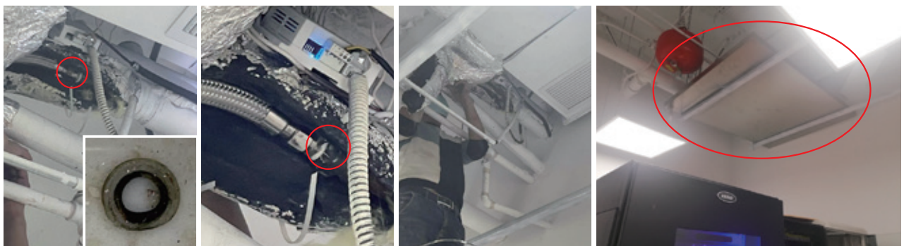
Packing that had deteriorated
